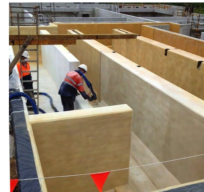
Concrete structures at Whitsunday Wastewater Treatment plant
