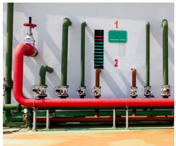
The red pipes denote fire hose supplies
