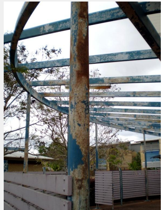
Galvanised steel and as waterborne coating system were erroneously chosen strictly on VOC criteria, without regard for long term durability, nor other more serious environmental impacts
