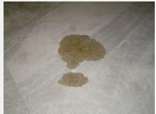
Oil stains and tyre marks on laitance-covered floor
