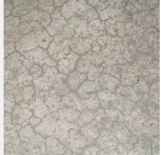
Laitance and shrinkage cracks
