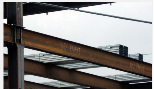
The fallacy that millscale itself can protect steel has been proved spectacularly wrong!
