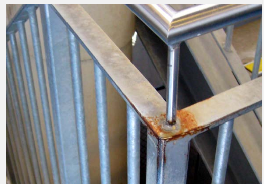
The highly reactive zinc layer of galvanized steel rapidly rusts when in contact with stainless steel.
